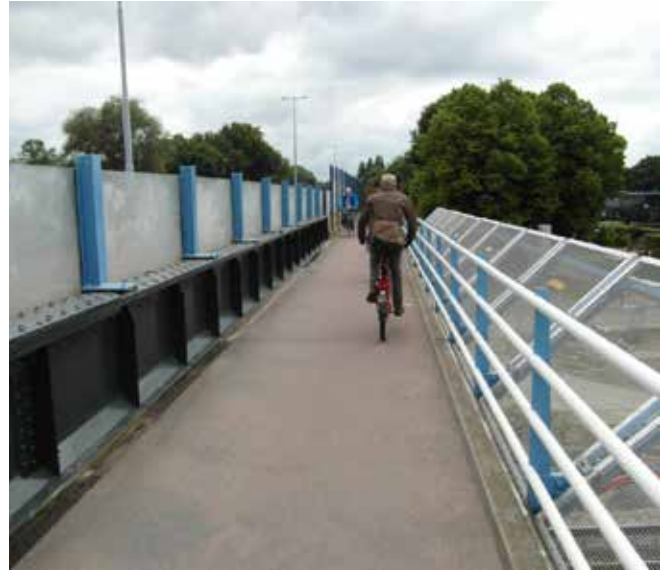
Utrecht - this narrow cycle-pedestrian bridge is part of a highway bridge (to left) over a railway corridor (to right).
